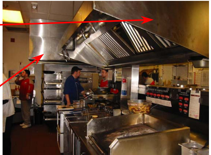
Figure 2. Exhaust Hood 1 and 2.
