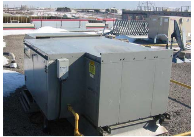
Figure 5. Direct-Fired MUA Unit.
